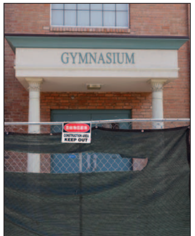
SCOTT CRABTREE/The Daily Sentinel The old Palisade High School is being torn down to make way for a new medical clinic.
